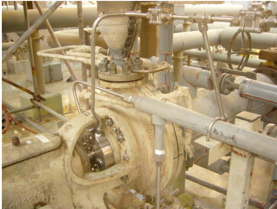
Figure 21: Perfectly operating mechanical seal with steam quench
