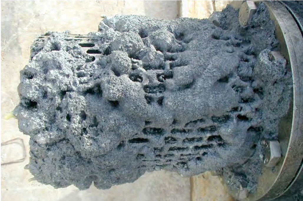
Figure 16: Clogged suction strainer
