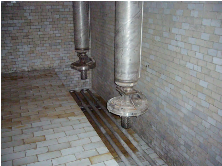
Figure 11: Installed pumps in a pit with side walls
